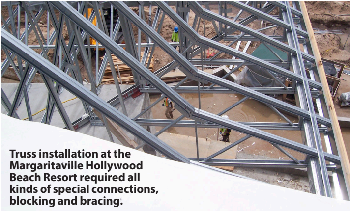
A cantilevered cold-formed steel truss design reflects the shape of a Polynesian-style roof by incorporating multiple truss system sections.
